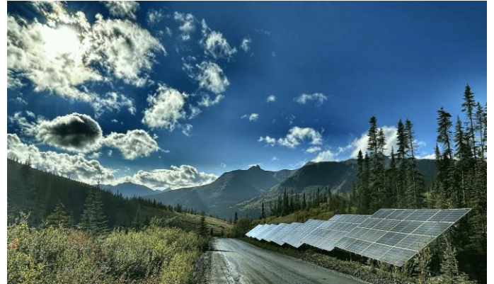
Solar panels at the Macpass Project leased through Tu Lidlini Petroleum |
